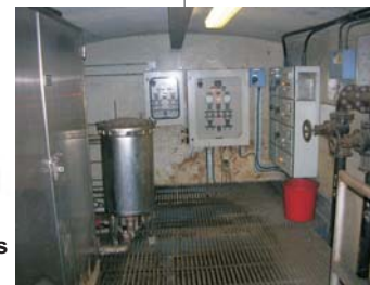
Tunnel Water Treatment Plants along MTR stations
