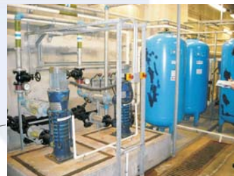
East Rail 400 Pumping Facilities
