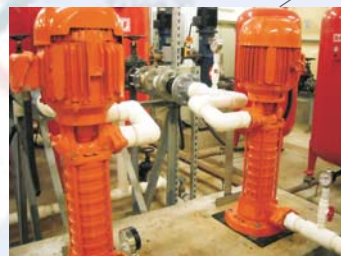
NAC 150 Pumping Facilities
