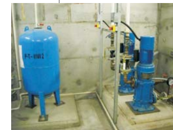
MOL 200 Pumping Facilities
