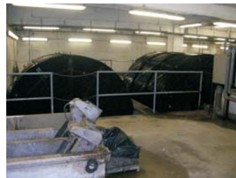
Sewage Treatment Facilities
