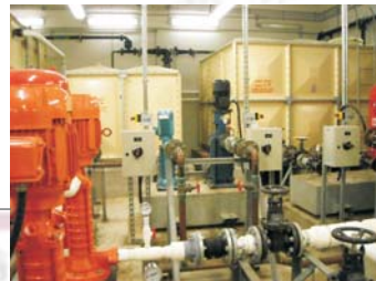
West Rail 450 Pumping Facilities
